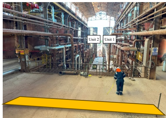
Figure 8. Existing Digestion area, with the orange rectangle indicating the location for KX Pilot between A1 and A2 of digestion units 1 and 2.
